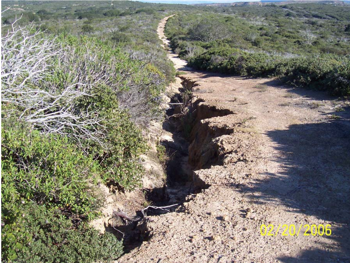
Picture 3: Rutted Section of Access Road
