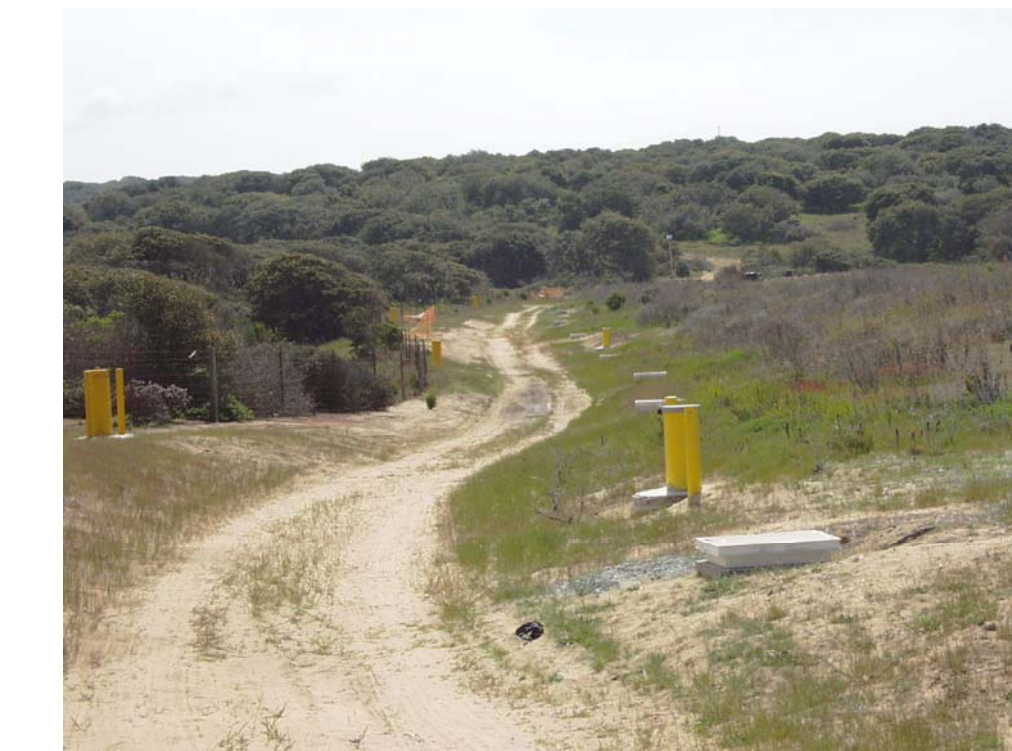
A line of extraction wells at the edge of Area F (to the right in the photograph) extracts landfill gas for treatment. Monitoring probes installed along the fence to the left show that the landfill gas in the soil at the property boundary does not exceed State standards.
