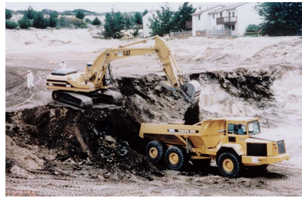
Excavation of wastes from Area A in 1996. The wastes were transported in trucks across Imjin Road and placed in the other areas of the landfill.
