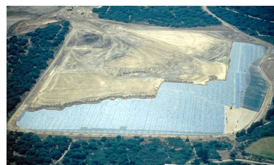
Construction of the engineered cover on Area F in 1998. Clean vegetative cover soil is being spread out over the geomembrane.
