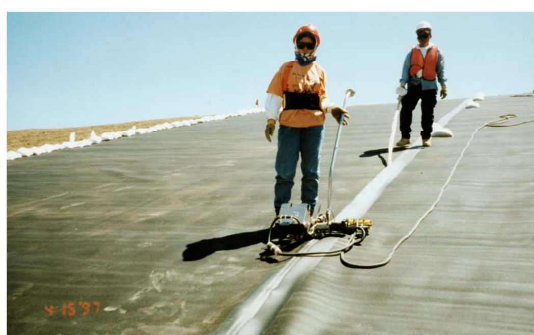
Geomembrane being installed on Area B in 1997. A special machine is used to weld together the adjacent seams to produce an impermeable layer within the cover.
