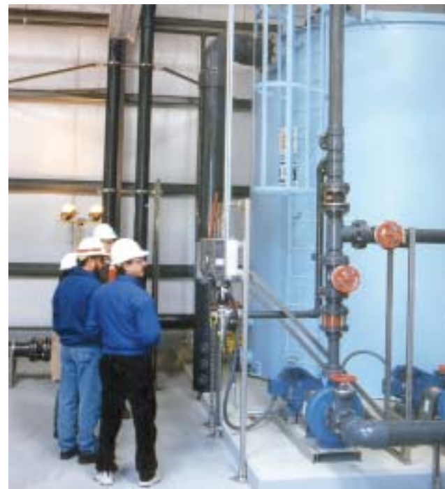
Engineers inspect the holding tanks of the 2/12 Groundwater Treatment Facility
