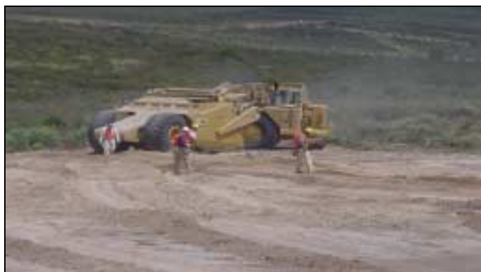
A UXO team searches for OE in soil removed from the Range 26 berm by the scraper in the background
