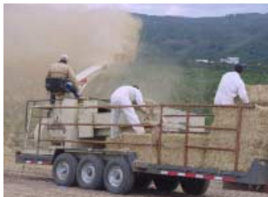
A site restoration crew sprays straw over a berm on the Del Rey Oaks site.
