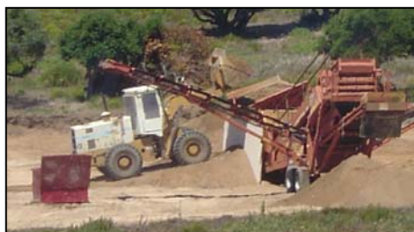
After scraping the Range 44 pad, the Army is now sifting the excavated soil.
