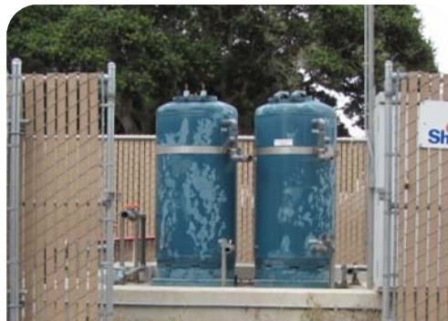
Off-Site System: Just like the other OU1 groundwater systems, groundwater is pumped through tanks that hold activated carbon. The TCE and other contaminants stick to the activated carbon in the tanks and are removed from the water. The clean water is then returned to the ground.
