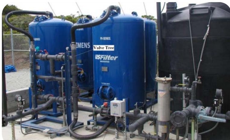
Northwest Treatment System: The OU1 groundwater is pumped through the blue tanks that hold activated carbon. The TCE and other contaminants stick to the activated carbon in the tanks and are removed from the water. The clean water is then returned to the ground.
