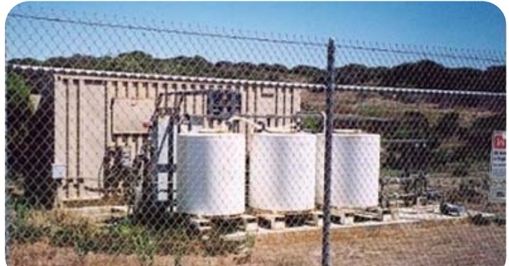
In the original system pictured above, the OU1 groundwater was pumped through the three white tanks that hold activated carbon. The TCE and other contaminants stick to the activated carbon. The clean water is then returned to the ground.
