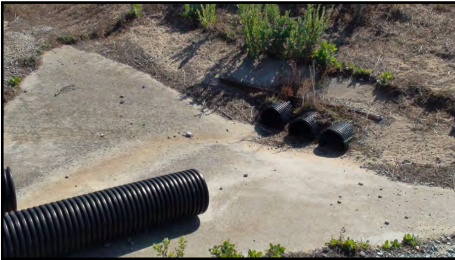
23. Phase 1 area downdrain catch basin (three 8-inch pipes), August 3, 2020
