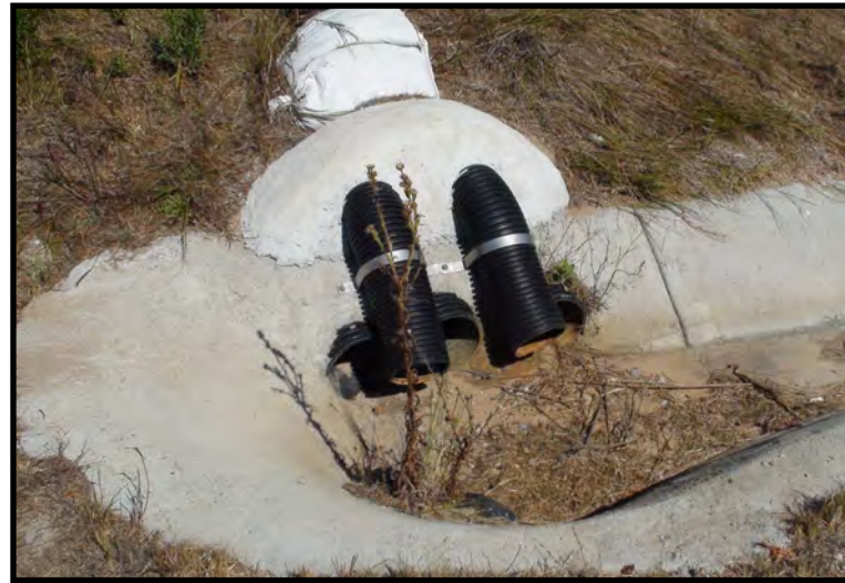
24. West side subdrain outlet (two 6-inch pipes) above and downdrain outlet (three 8-inch pipes) below, August 3, 2020
