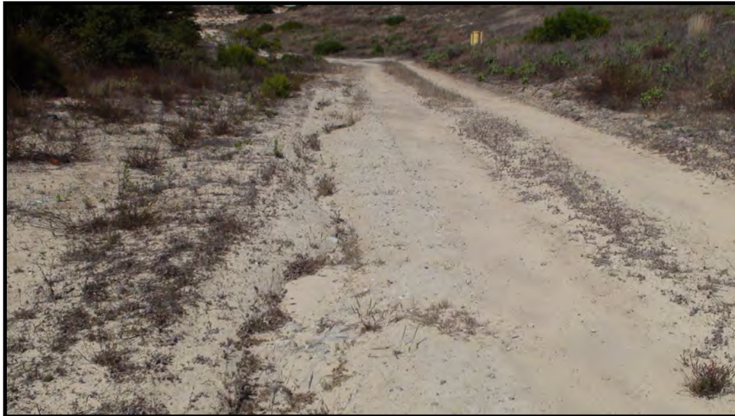
80. Perimeter service road erosion rills, viewed from southwest Area F facing north (August 3, 2020)
