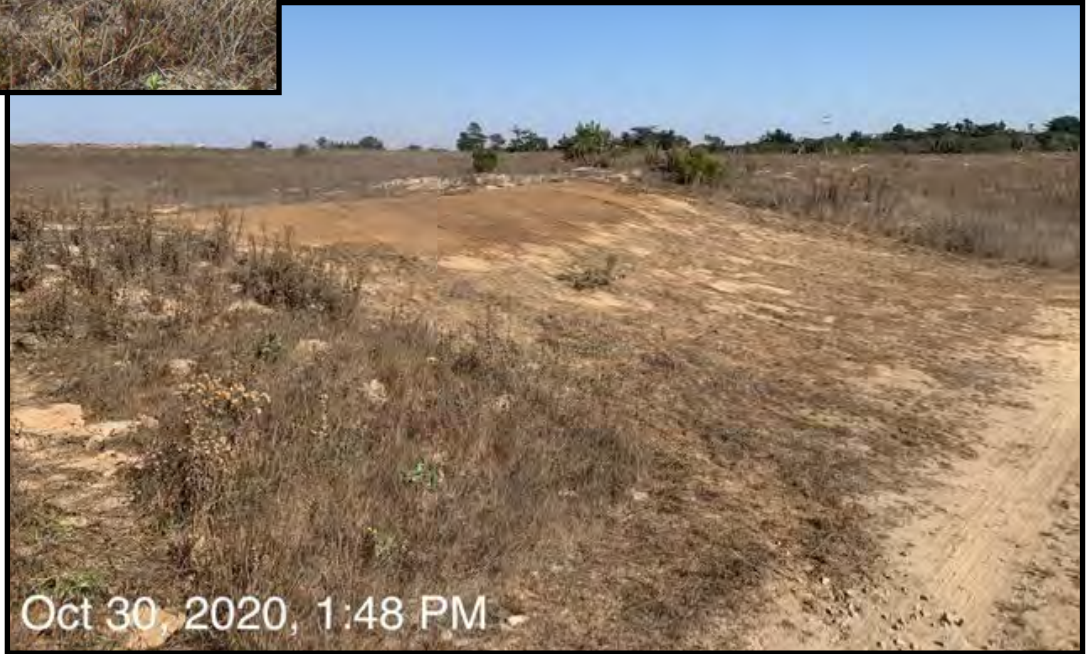
33. Repaired berm on south side of Area F, facing east from perimeter road (October 30, 2020)
