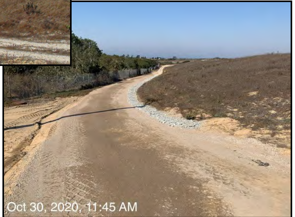
77. Perimeter service road repaired with rolling dips and rock-lined drainage swales, southwest Area C facing northwest (October 30, 2020)
