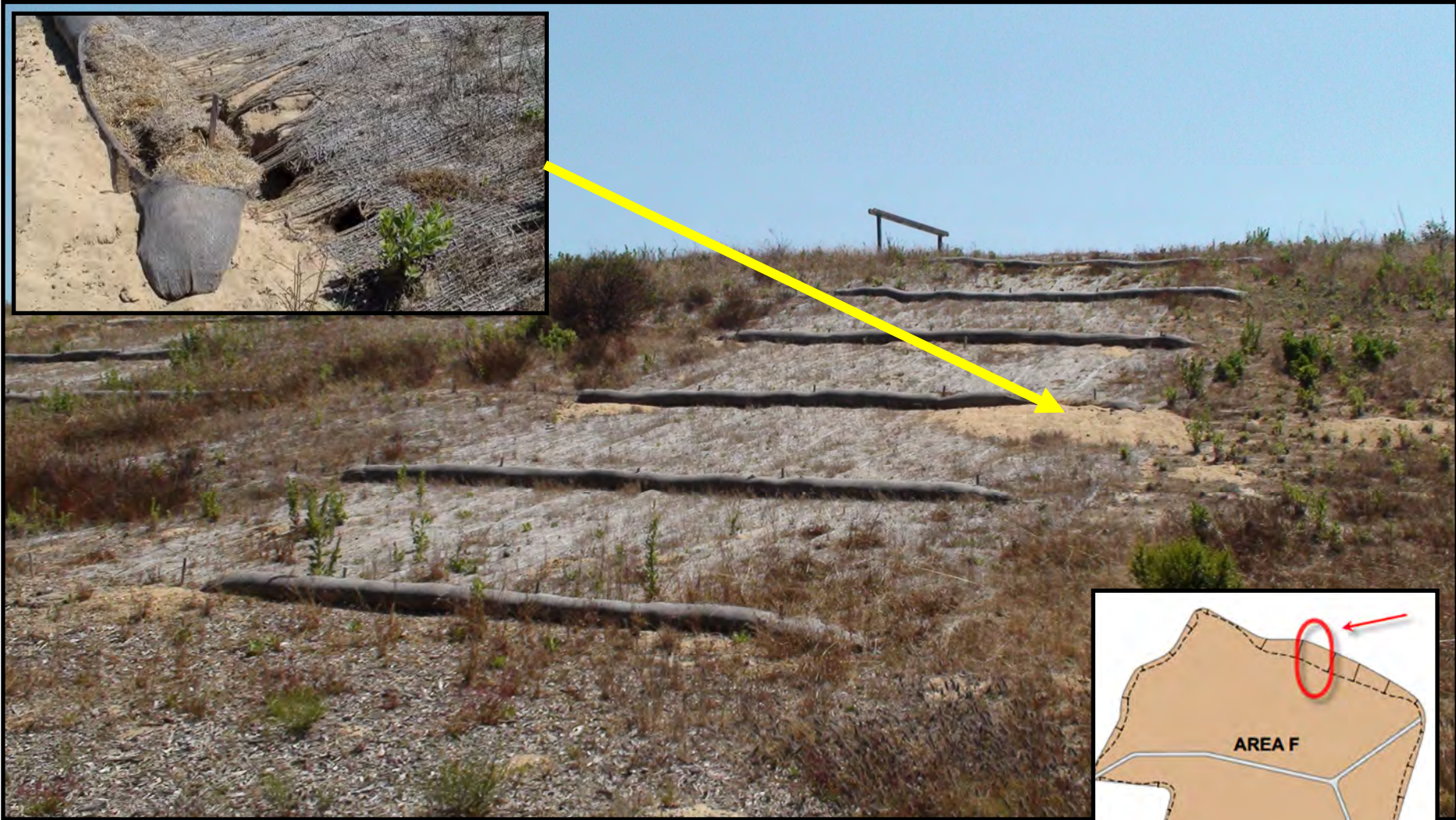
Area F north slope repair area with animal burrows (August 3, 2020)
