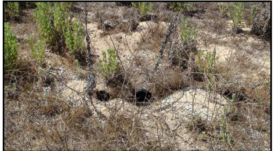
16. Downdrain outlet (two 8-inch pipes) on east side of Area D (August 3, 2020)
