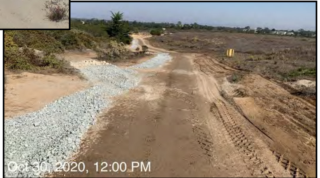
81. Perimeter service road repaired with rolling dips and rock-lined drainage swales, viewed from southwest Area F facing north (October 30, 2020)
