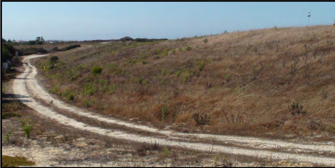
76. Perimeter service road with erosion rills, southwest Area C facing north (August 3, 2020)
