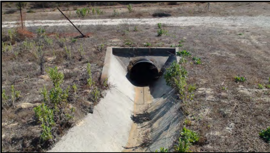
44. Area E northern V-ditch outlet to infiltration basin (August 3, 2020)
