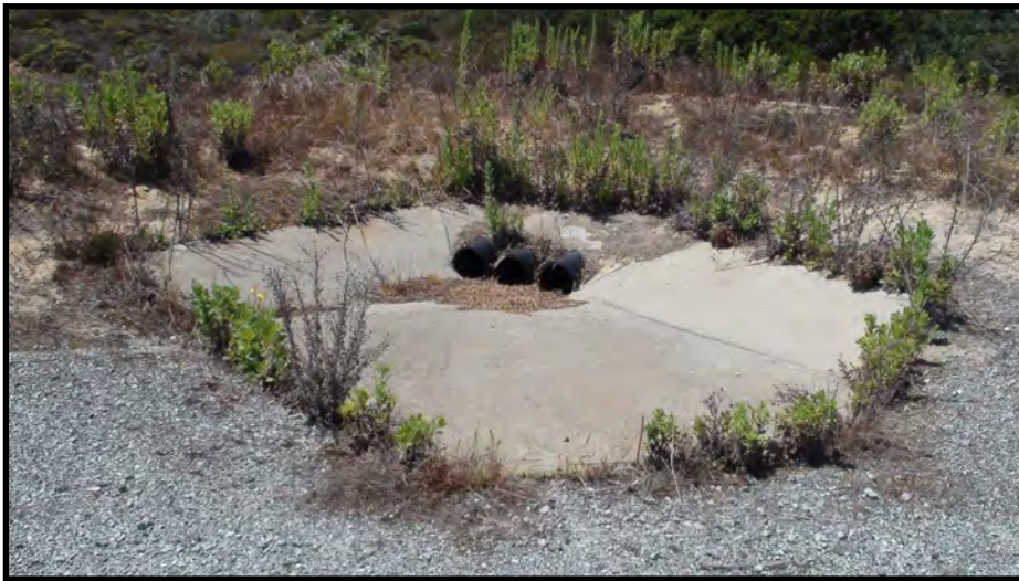
13. Downdrain inlet (three 8-inch pipes) on west side of Area D (August 3, 2020)
