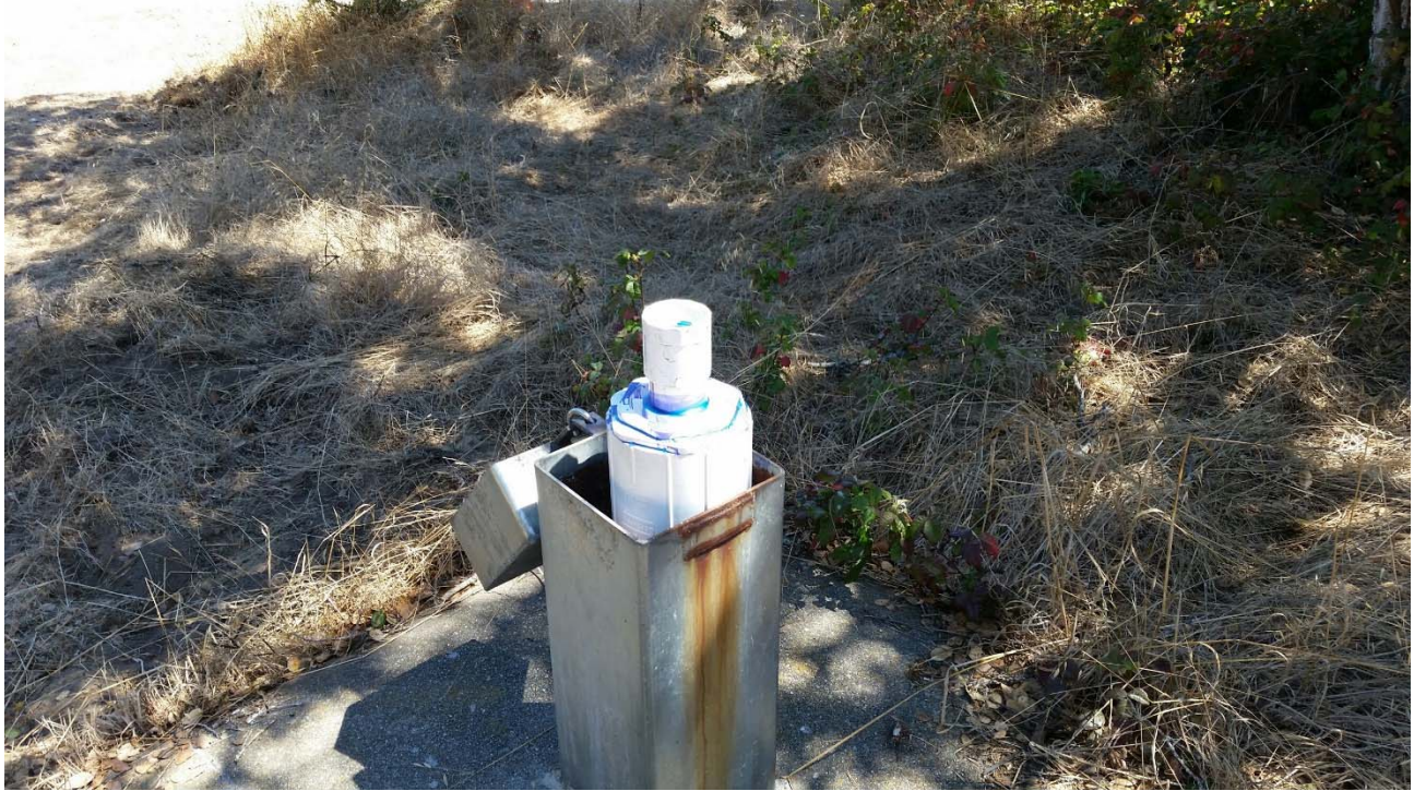
Photo 02 – Wellhead fitting used to connect to air compressor after a well has been filled with grout.
