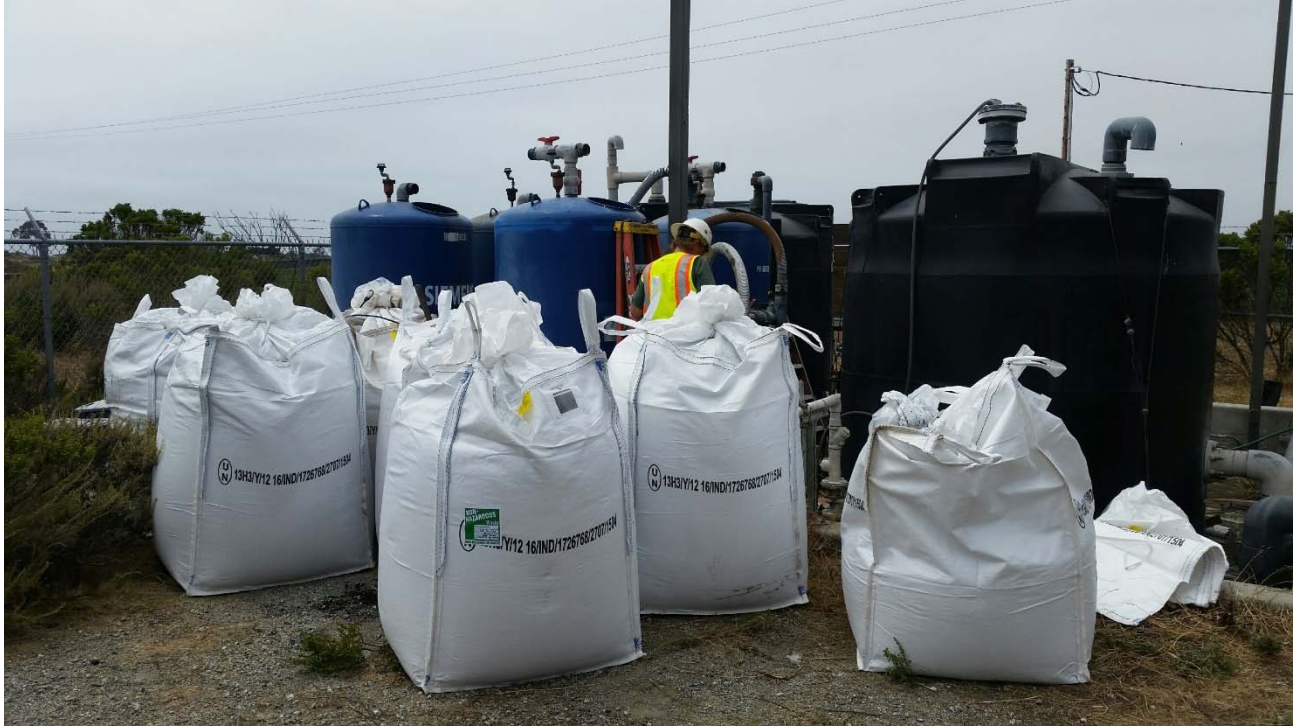
Photo 03 – Seven super sacks of GAC removed from vessels.
