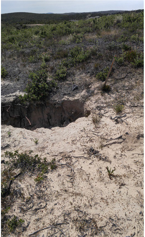
Photo 2: Erosion Monitoring Location (see Figure 2)
