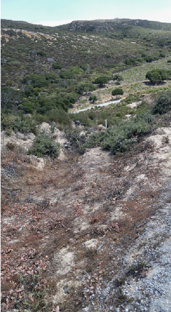
Photo 1: Erosion Area 1 (see Figure 1)
