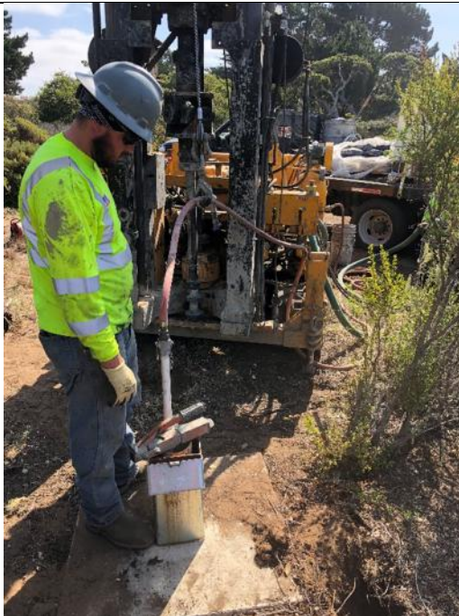
Description: Using a tremie pipe to pump the grout to the bottom of the well at MW-OU2-60-A.
