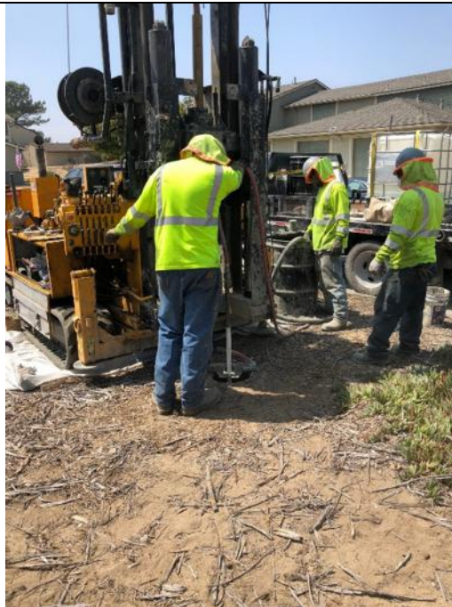
Description: 95% Portland Cement / 5% Bentonite is mixed and Pumped in the well with a tremie pipe at MW-BW-64-A.
